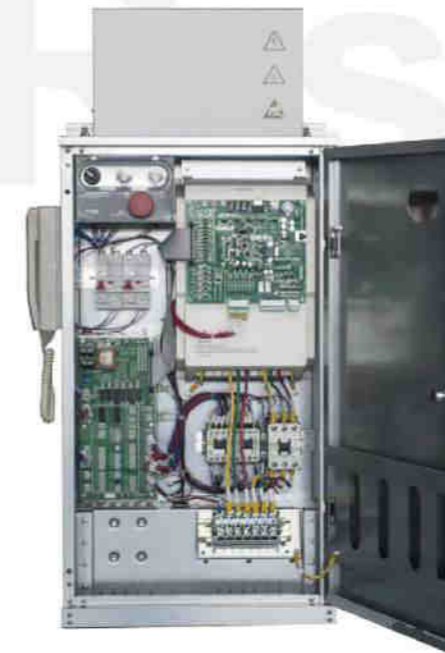
Machine room 机房
